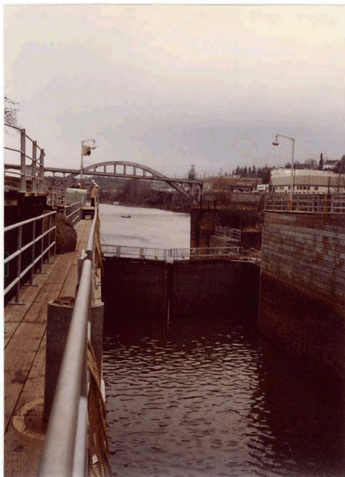
Gate No. 1 Willamette Falls Lock
