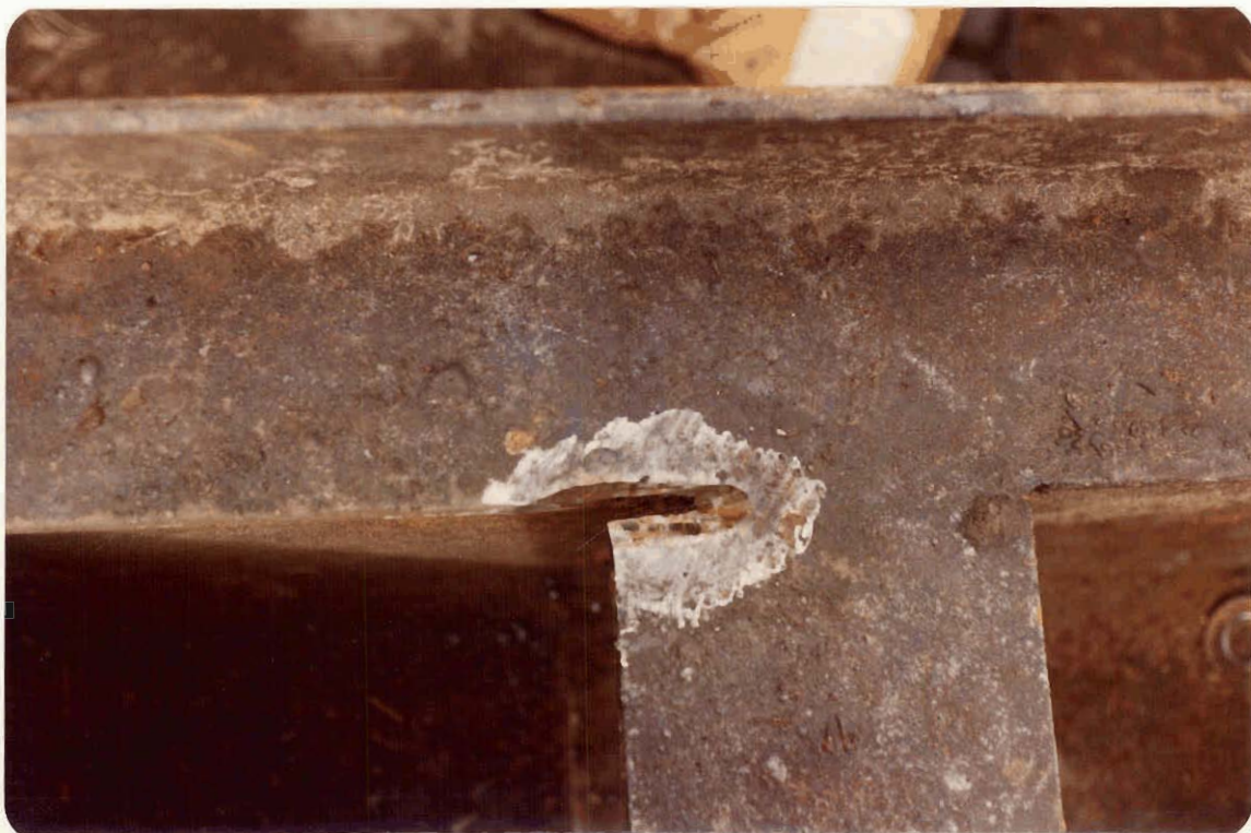
Frame (12) 5 May 82 Gate No. 1 Gouged crack Left Leaf
