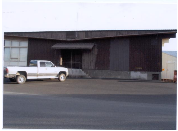
High School Addition, faded, old paint.
